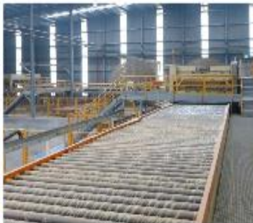
Roller conveyor to board turner
