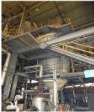
Chip washing plant
