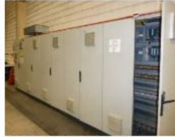
MCC's, Siemens S7 control
