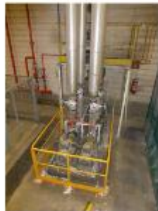
Secondary heating circuit
