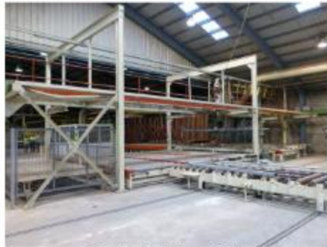
Conveyors for finished board stacks
