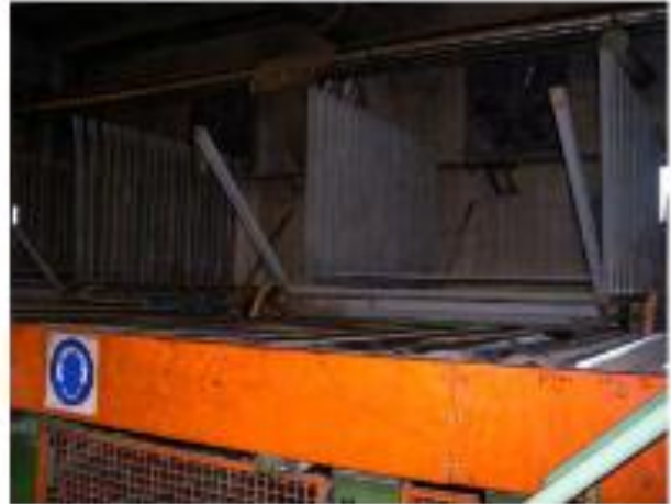
Board cooling turner
