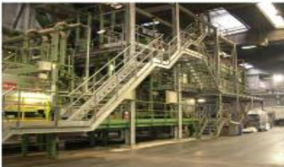
Forming station Dieffenbacher
