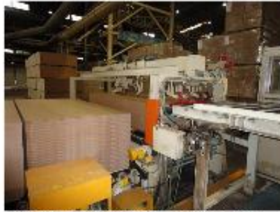
Destacking station with infeed pusher
