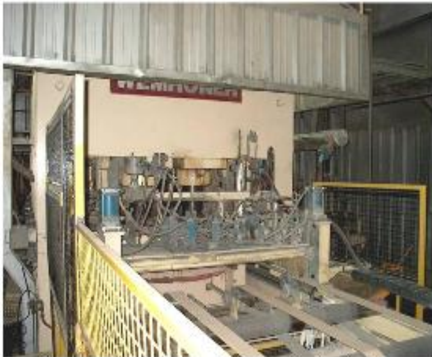
Press unloading conveyor & press unloading device
